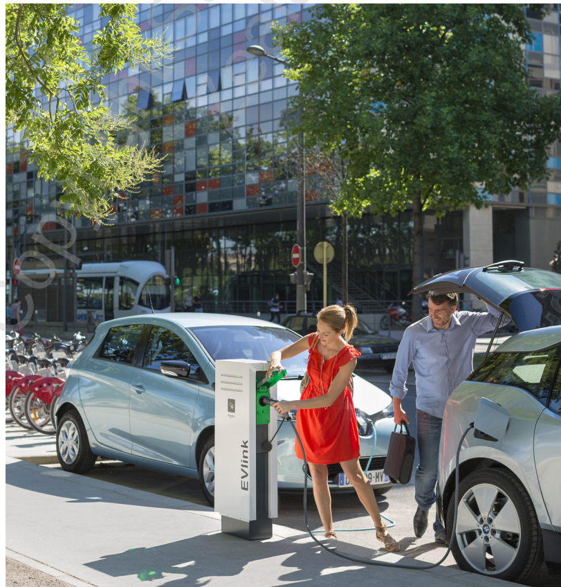
Figure 12 – Mode 3 (AC) 22 kW three-phase charging station
